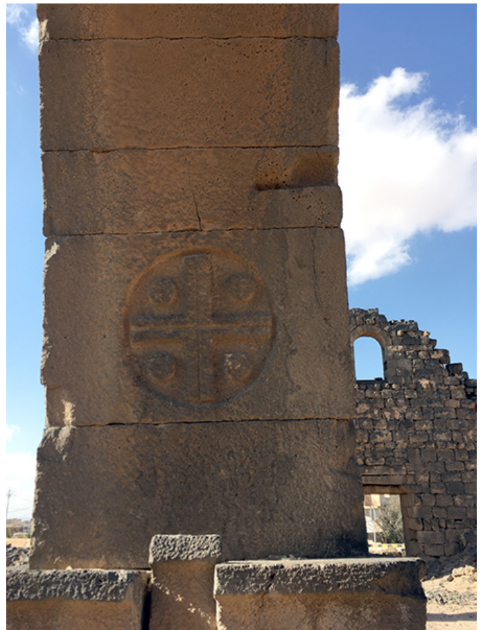
Fig. 4: An "Umm el-Jimal cross" carved into the pier of an arch of the Western Church, Umm el-Jimal. (Photo courtesy of Elizabeth Ursic.)
